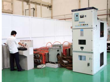
▲ Temperature rise test
